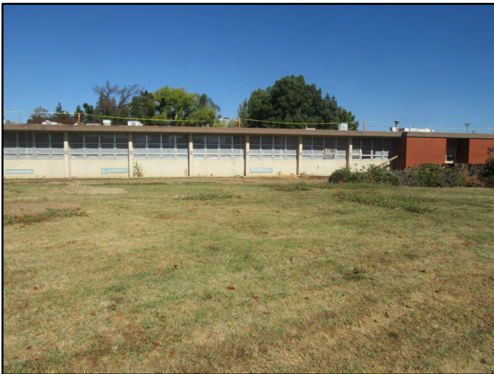
Manicured lawn south of Mohr Hall in the south part of the site, looking north; 10/16/18. Demolition of Mohr Hall has begun.
