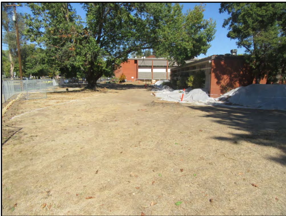
Trees and dirt area west of Mohr Hall, looking north from the southwest corner of the site; 10/16/18. Demolition of Mohr Hall has begun and a few trees have been removed.
