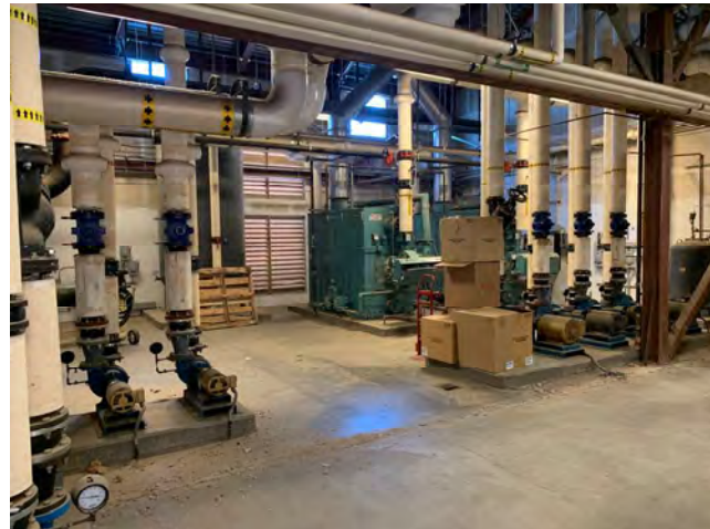
FLC Central Plant Upgrade
