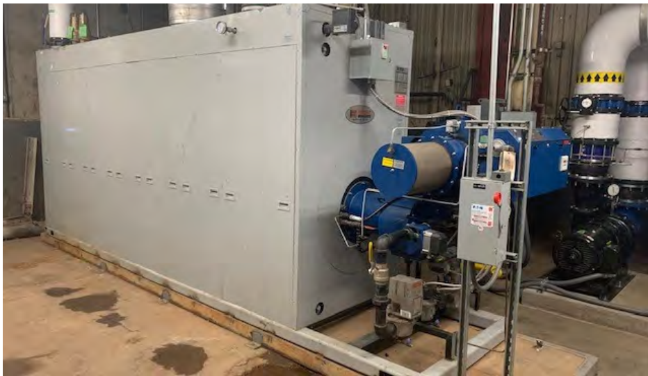
New boiler unit
