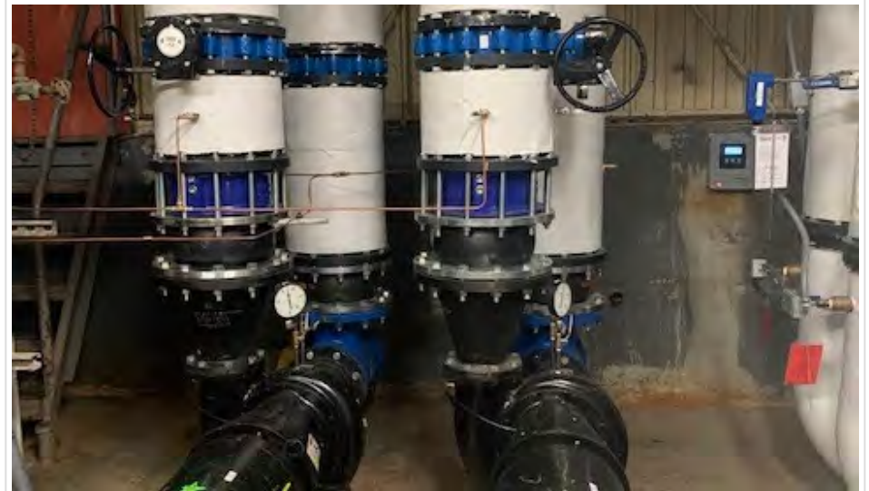
New hot water valves
