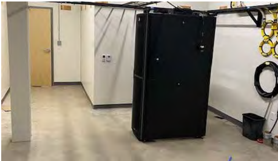
Existing MDF from North
