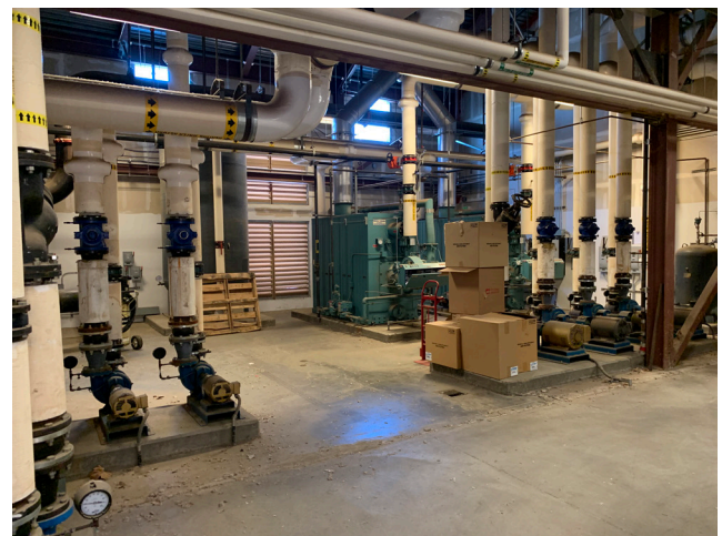
FLC Central Plant Upgrade
