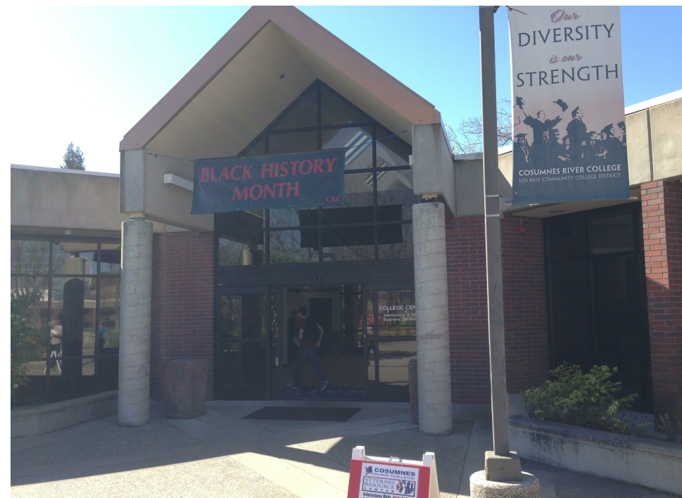
4 COLLEGE CENTER EXTERIOR: REMOVE (E) CONC COLUMNS & FOUNDATIONS BELOW; REMOVE (E) BEAMS, LIGHTING, ROOF TO EXTENT INDICATED ON ROOF DEMOLITION PLAN; REMOVE (E) LANDSCAPE ELEMENTS
