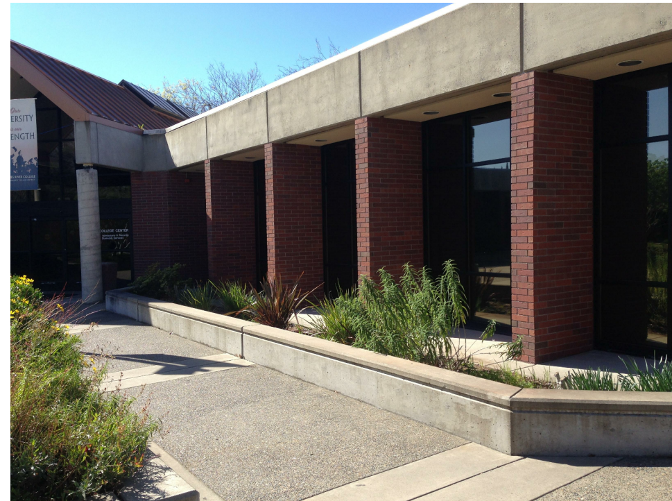
5 COLLEGE CENTER EXTERIOR: REMOVE (E) CONC FASCIA, CEMENT PLASTER SOFFITS, LIGHTING; REMOVE (E) CONC SEAT WALL
