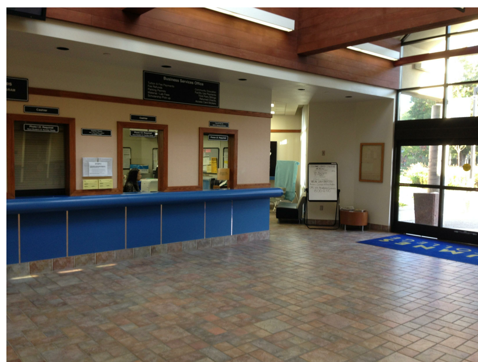
1 COLLEGE CENTER SERVICE WINDOWS: BASE BID: REMOVE (E) LAMINATE SKIRT, WALLCOVERING ABOVE COUNTERTOP, WOOD TRIM, SIGNAGE ADD ALT #X: BASE BID PLUS REMOVE (E) BULLNOSE COUNTERTOP, SERVICE WINDOWS
