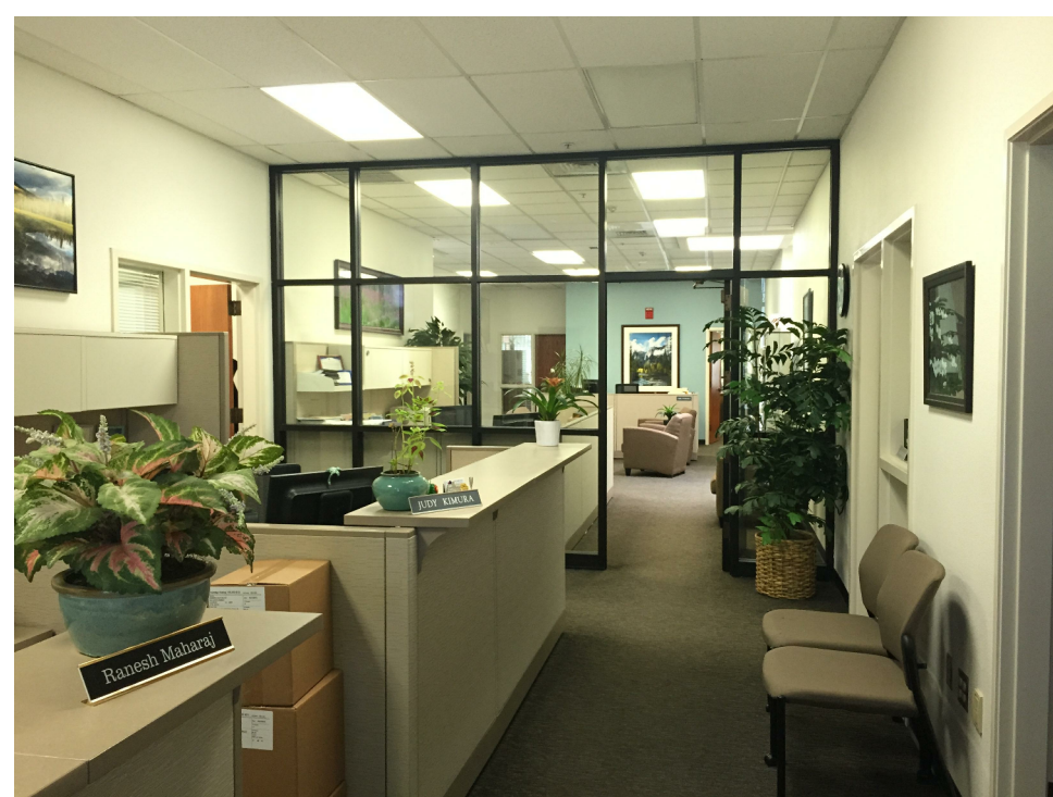
3 COLLEGE CENTER OPEN OFFICE: REMOVE (E) ALUMINUM STOREFRONT PARTITION; REPAIR ACOUSTICAL CEILING GRID AS REQ'D.
