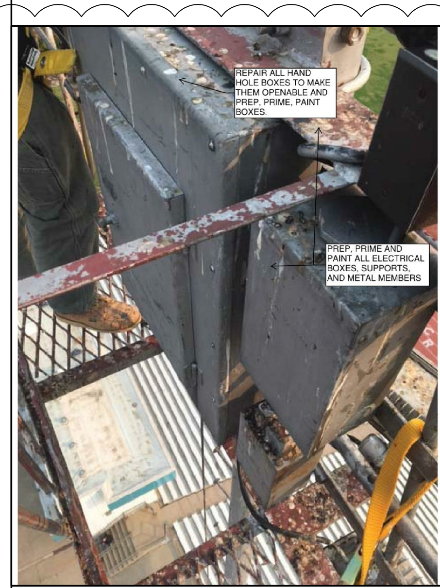
SUPPORT PLATFORM AND HAND HOLE BOXES AT TOP OF LIGHT POLES
